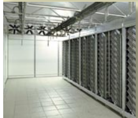
No suspended ceiling and rails in floor for easy cleaning
