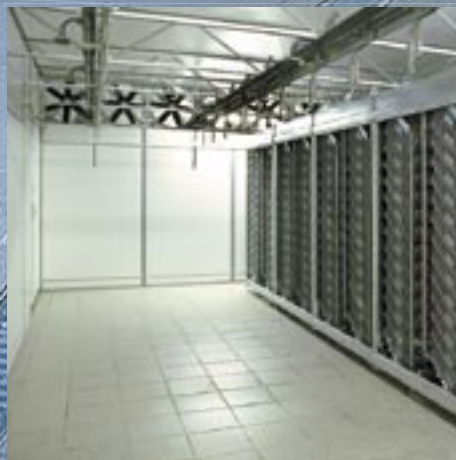
Inside view from setter
